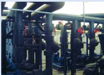
Armaflex tube used to insulate a large plant room
